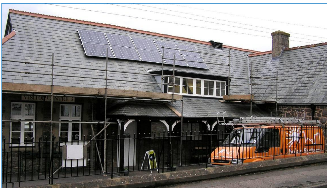
Solar PV panels erected on the Porlock Visitor Centre (ENPA)
