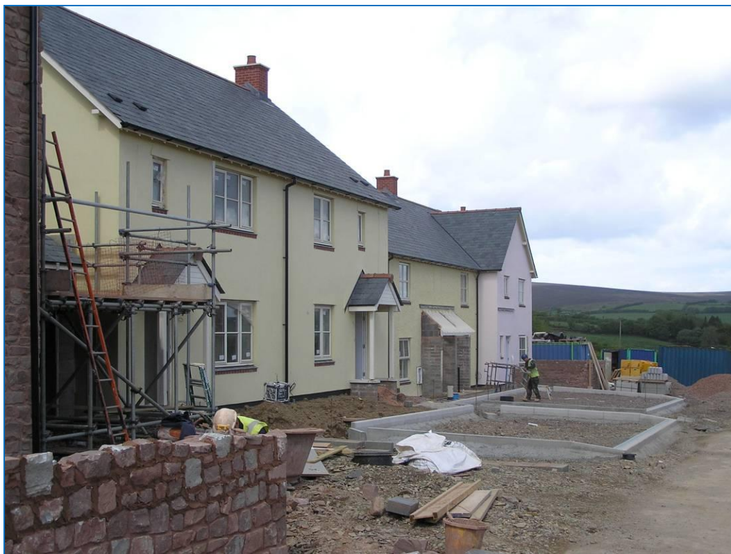
New housing under construction at the Cutcombe Market Site – Wheddon Cross (ENPA)
