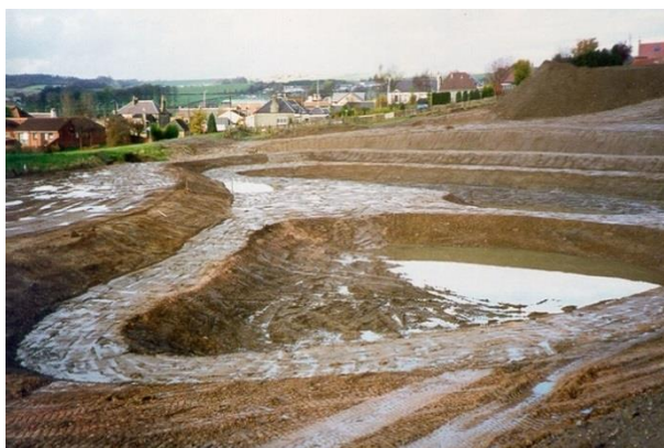
Figure 13: care needs to be taken during the construction of SuDS to ensure that the receiving environment is protected from sediment-laden surface water runoff. Credit: Susdrain (2016).
