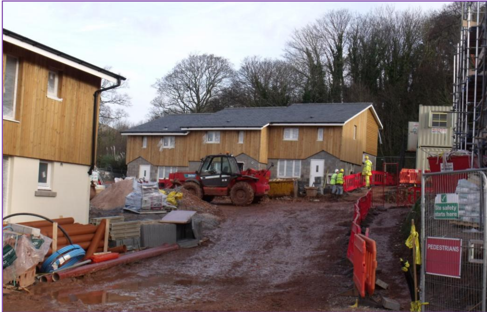
© ENPA – New local affordable housing under construction in January 2013: Villes Lane Porlock
