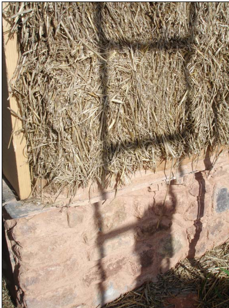
Figure 9. Detail of straw bale wall construction for new build straw bale houses at Raleghs Cross, Exmoor.
