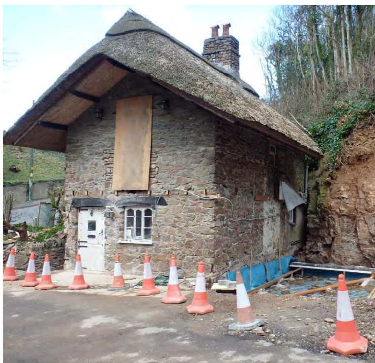
Work in progress on an extension to provide an additional bedroom at Royal Castle Lodge, Castle Hill, Lynton
