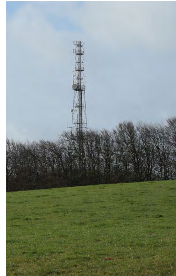
Elworthy phone mast
