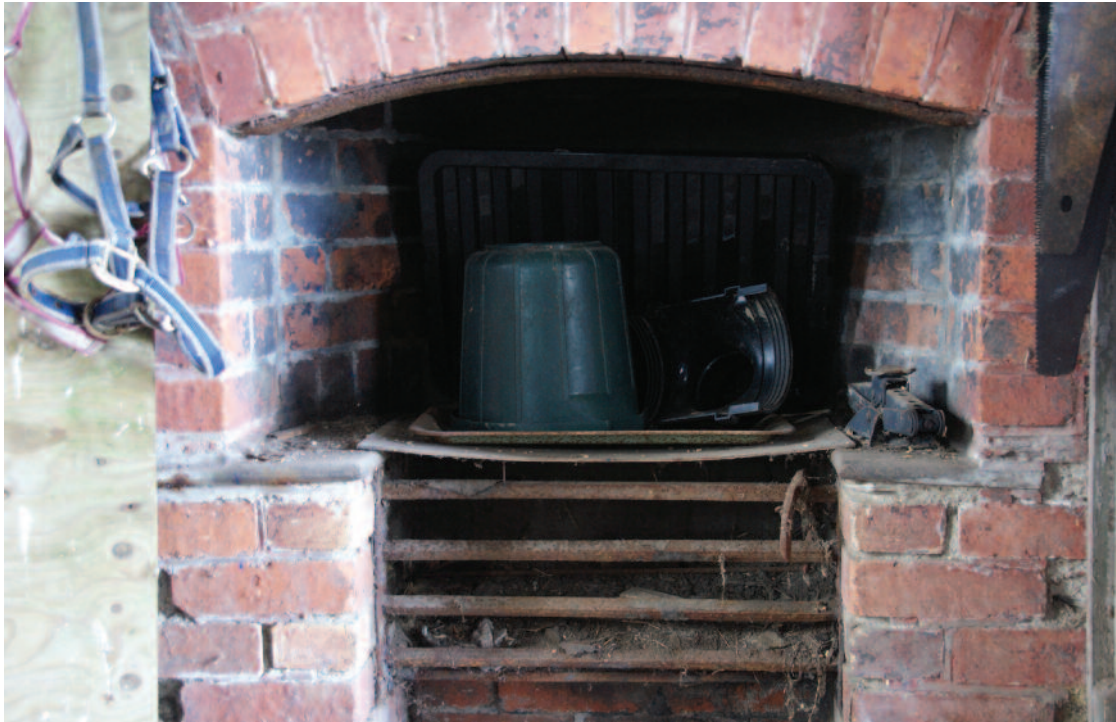
Range with iron frontage located in Room 2, western wall (Photo Nicholas Dawson July 2011)
