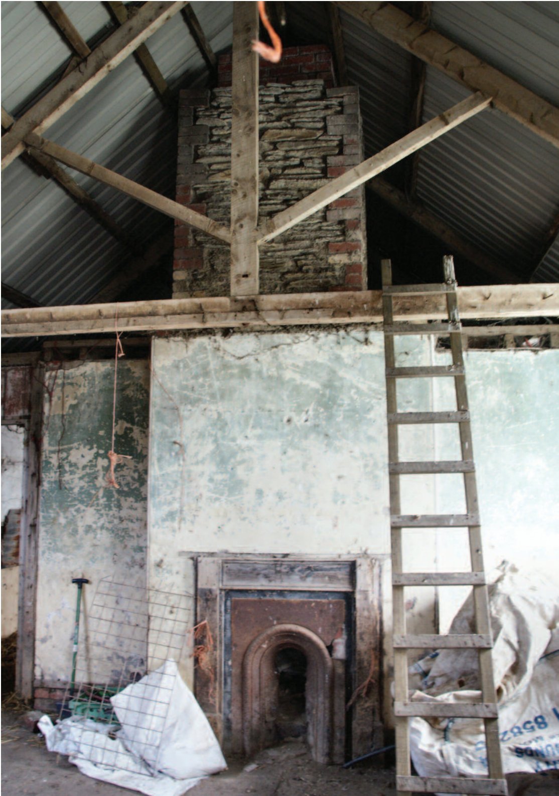
Cast iron fireplace and stone with brick quoined chimney stack located in Room 2, eastern wall (Photo Nicholas Dawson July 2011)
