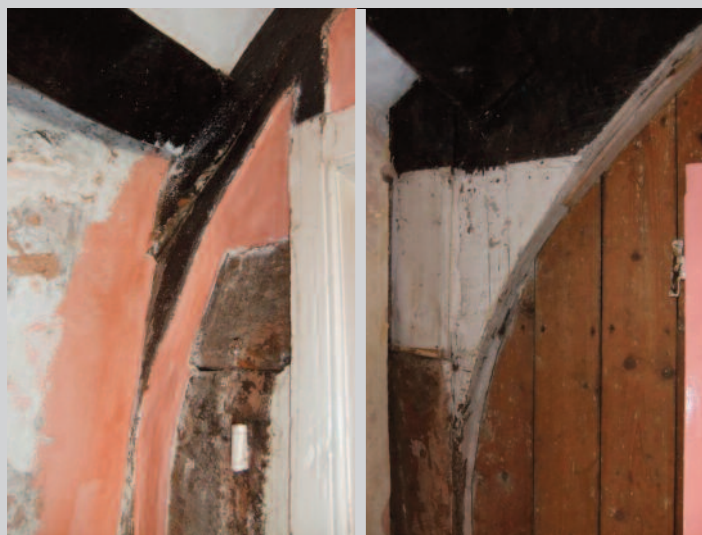
Left: Part of jointed cruck frame with part of an early door frame to a solar. Right: True cruck frame in same house.
