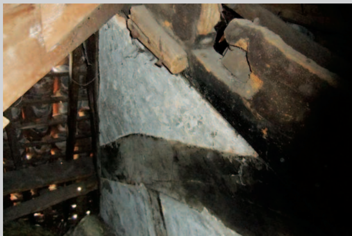
A house with smoke blackened roof timbers in West Street. Seen here is a jointed cruck frame with rod and daub infill.
